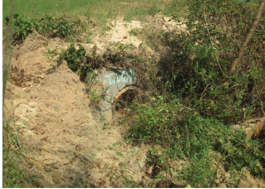
Photo: Grass Clippings Dumped Around Storm Sewer
