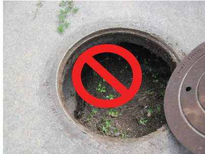
Clippings Dumped in Storm Sewer!
